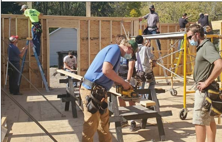
Building Trades instructor Kale Skogen supervises as the high school students work on house 76.
